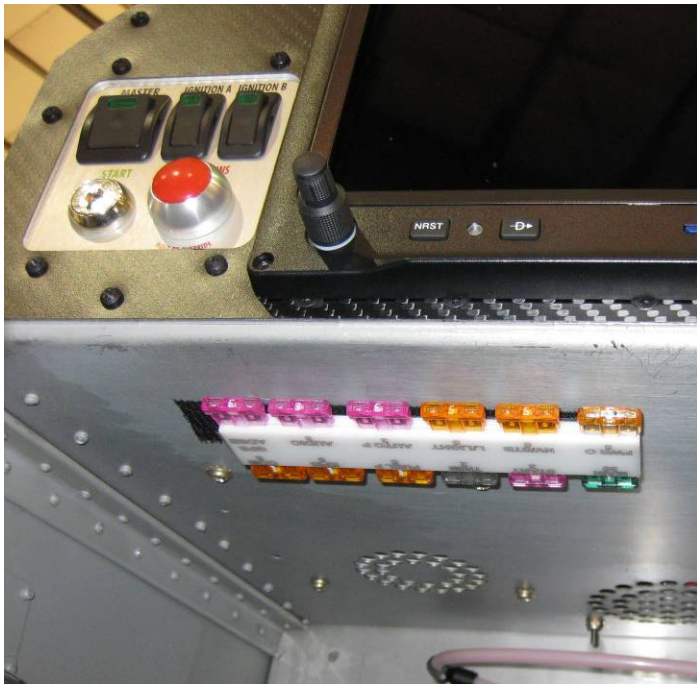
FUSE HOLDER UNDER PANEL
